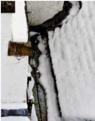
Heat trace wire on castle roof
